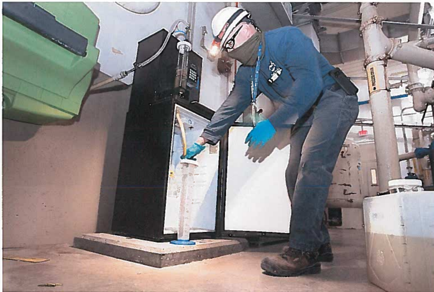
Lead operator Jason Chou collects a water sample at the West Boise Water Renewal Facility, Thursday, Aug. 13, 2020. Samples are taken at various stages in the wastewater renewal process and tested for COVID-19.
