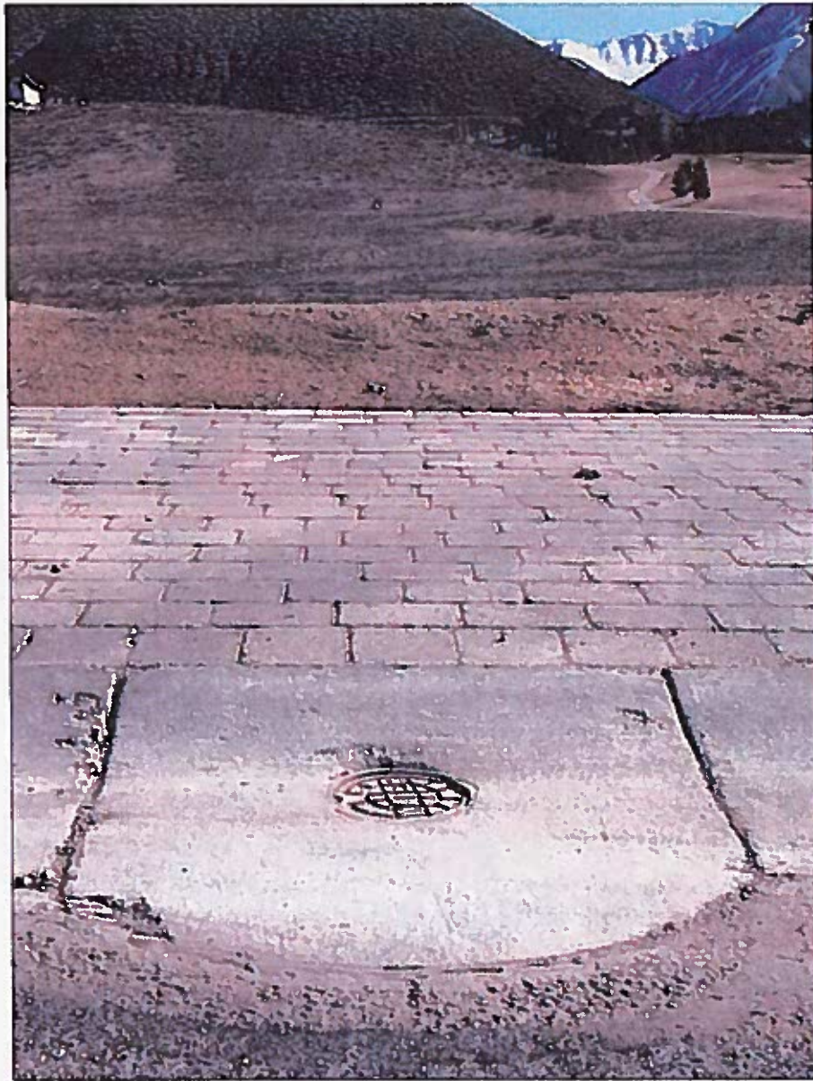
Example of stubbed in service main
